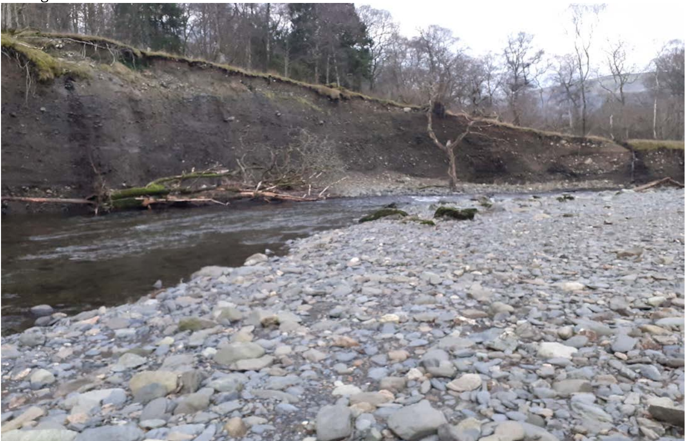
Damage to River bank and the River bed ...
