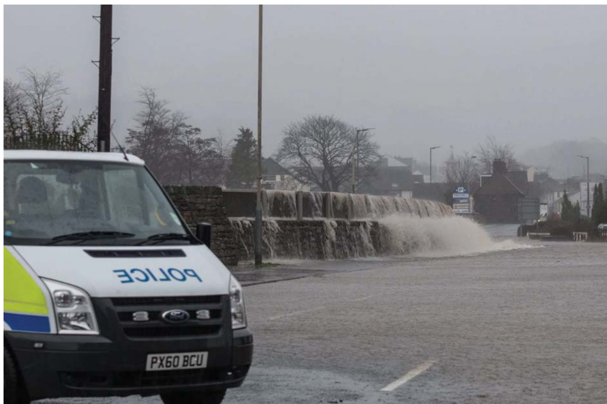
Figure 13: Compromised river defences 2015
